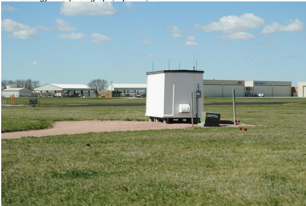
Fig 11. View of utilities infrastructure near southwest end of Runway 13-31, looking south. Tallgrass Archaeology LLC photograph, April 11, 2024.
