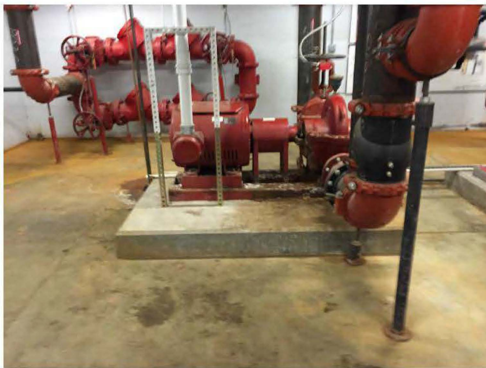
Photo 5: HEF discharge system inside Building 261 – Main Hangar (former location of AFFF storage)
