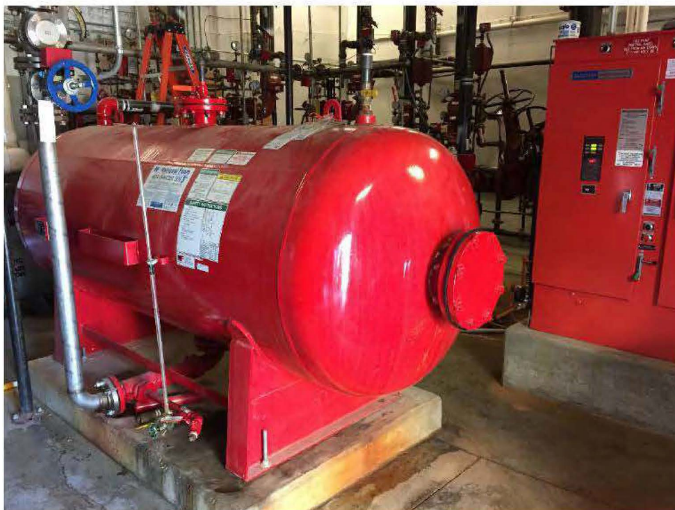
Photo 10: AFFF storage tank in Building 241 – ANG Paint Facility
